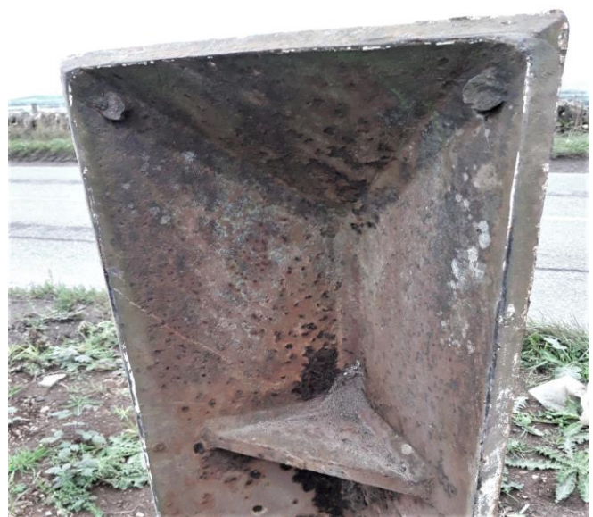
Pictfield milepost: View of the hollow rear of the milepost showing the triangular brace that has been welded to provide extra strength.
